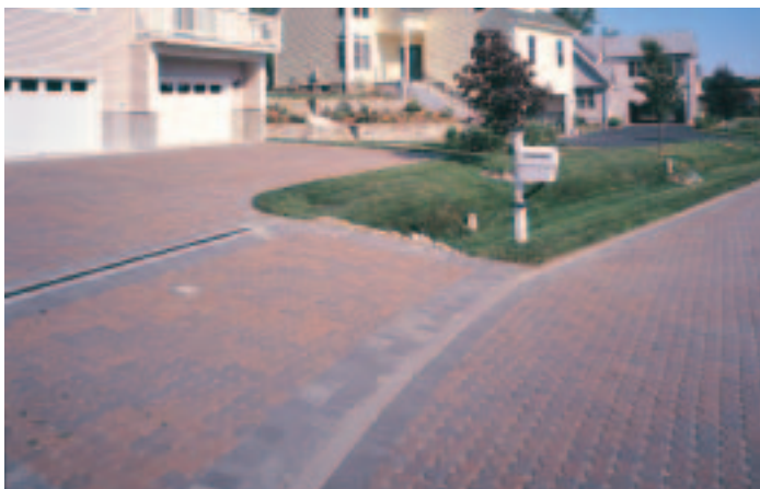
Figure 2. Slot drains at the ends of the PICP driveways facilitated sampling and collection of runoff.
