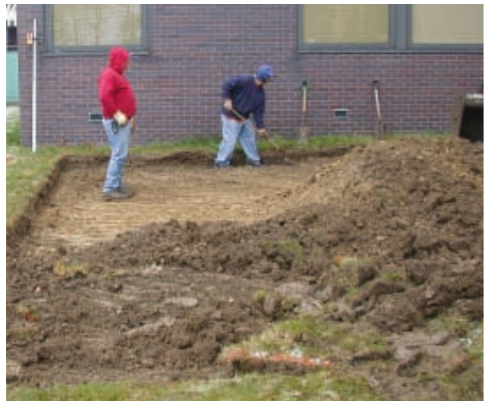
Figure 5. A clean excavation cut in the soil may need some touching up with a shovel to create perpendicular sides.
