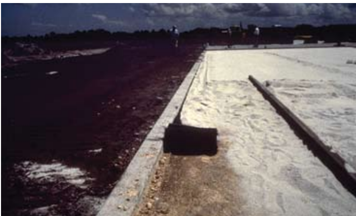
Figure 8. Woven geotextile contain bedding sand from migrating into curb joints or between the curb and base.
