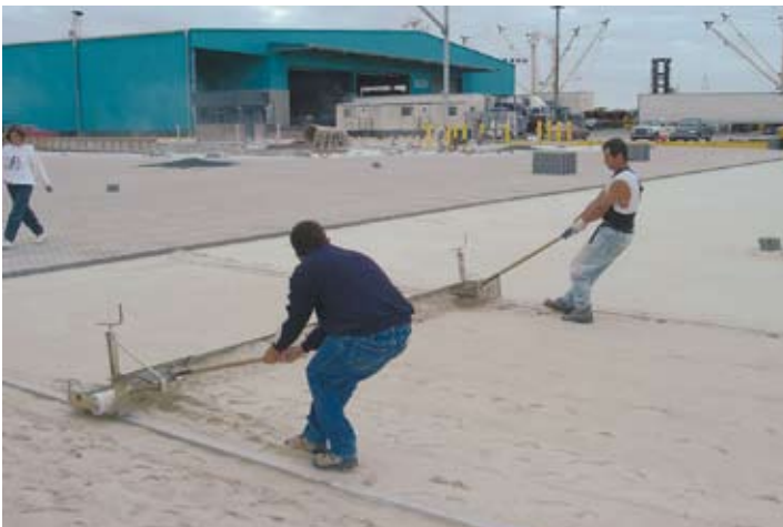
Figure 5. A two-man, hand pulled screed can level large areas of bedding sand. This is a port paving project in Florida.
