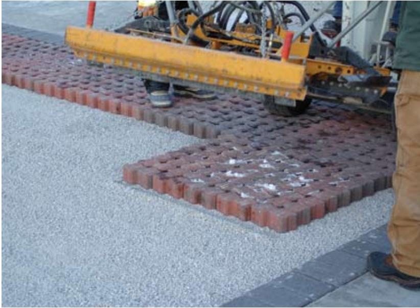
Figure 5. The permeable interlocking concrete pavers are supplied and installed in layers on the screeded bedding material, pea-sized aggregate (bedding sand is never used in PICP). Note the snow on the pavers doesn't interfere with installation and the border course against the concrete curb provides a finished edge.
