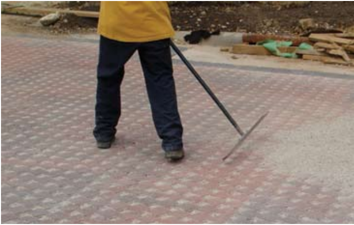
Figure 8. The paver openings are filled with the small stones (CA-16) and excess stones are removed from the paver surface prior to compaction.
